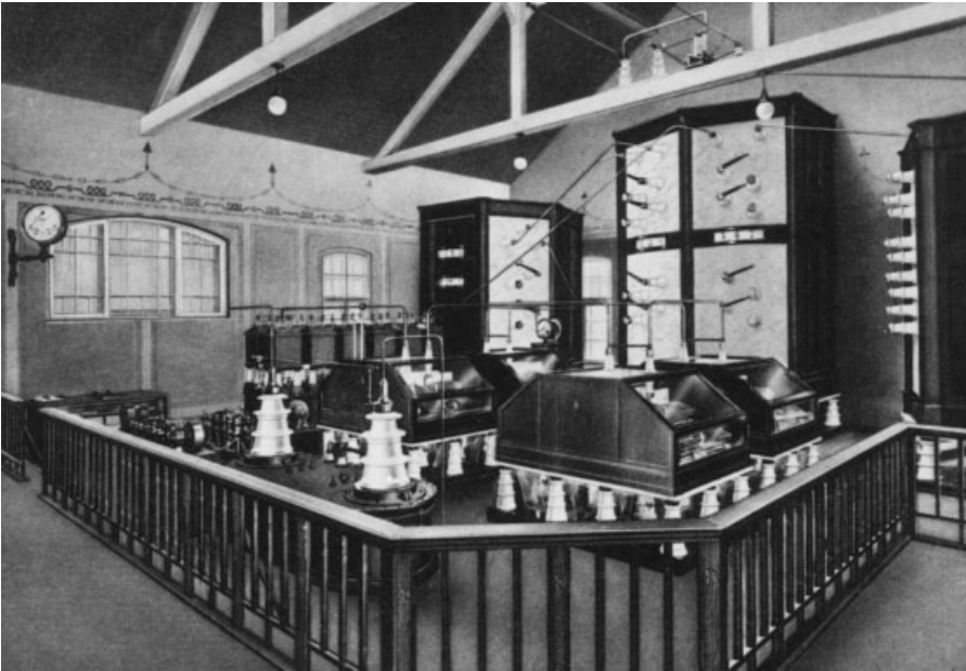
Figure 17.5 Transmitter room of the radio station at Nauen, Germany, around 1914. (Courtesy of Siemens Press Photo.)
