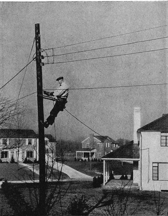
Installer connects a drop wire to provide service for a new telephone subscriber.
