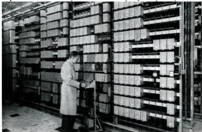
— 2000 Type Equipment racks
