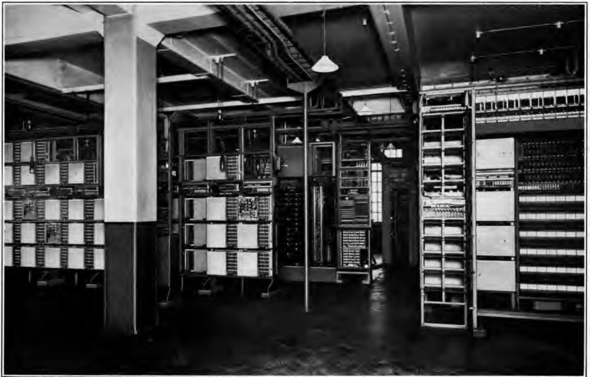
Archway Exchange, London—General View.
